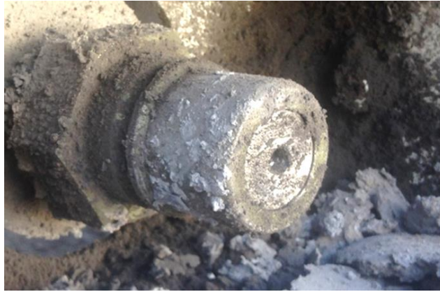
Figure 18 - Example of a Contaminated Receiver - No Dust Cap Fitted
