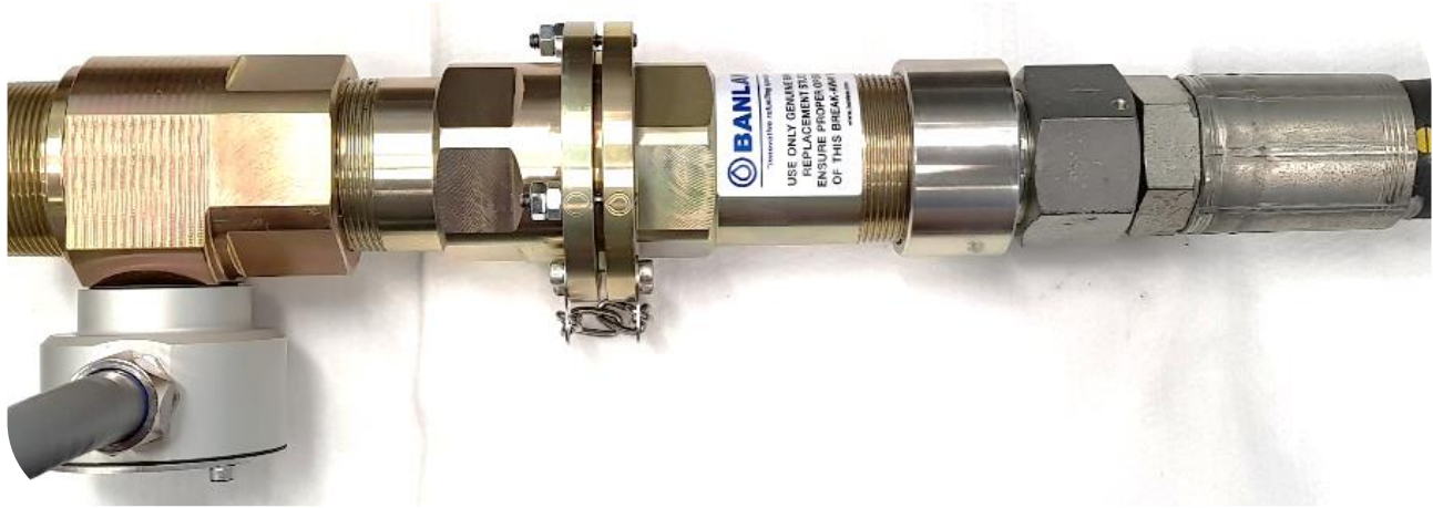
Figure 26 - FuelTrack BAV Installed
